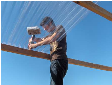
Daniel secures a panel of piping on a stall. Six 12'-long panels drilled into the framework.
